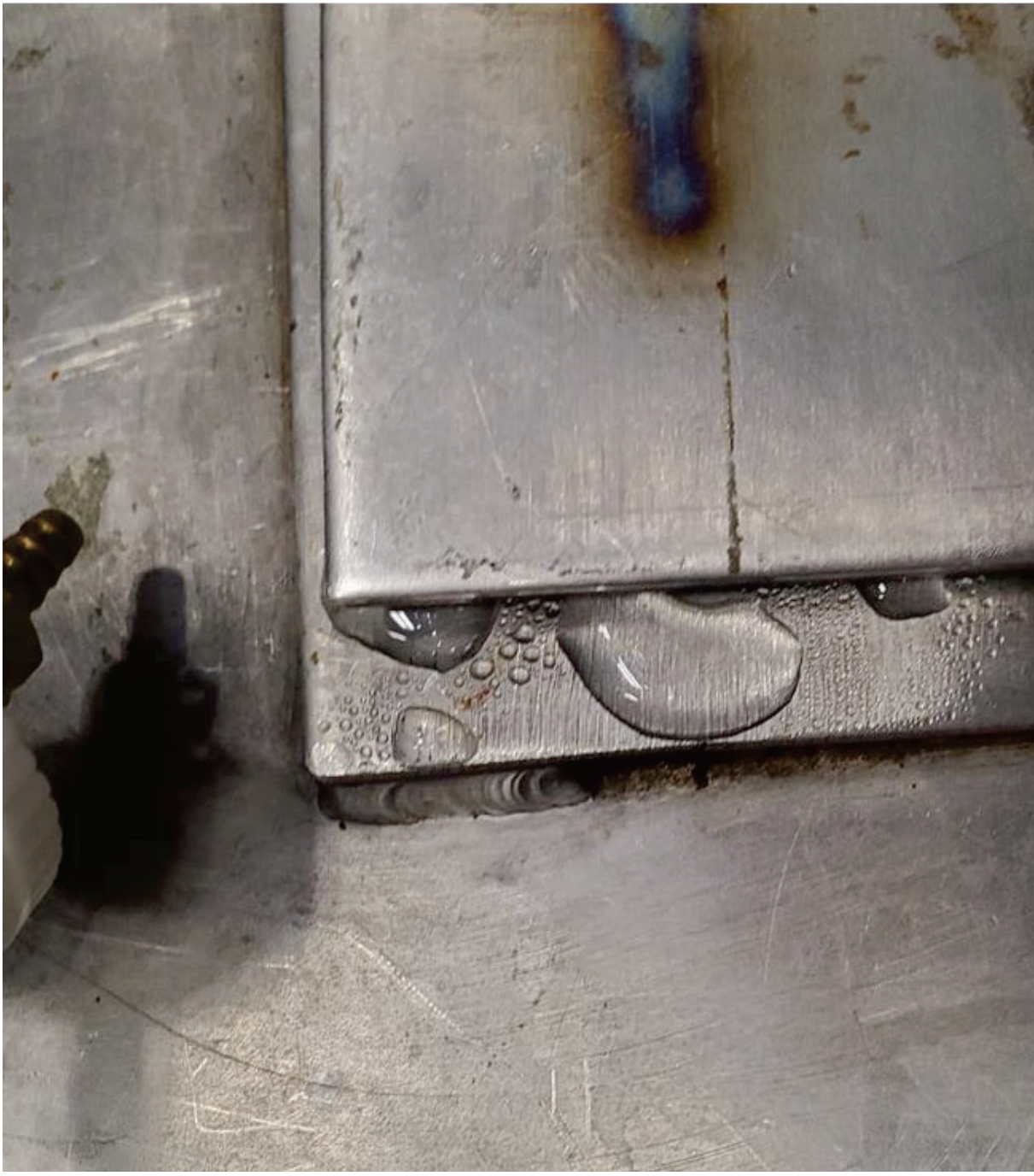
Figure 1: Condensation at threshold of 20B-TK-1 hatchway opening observed during field response actions:
