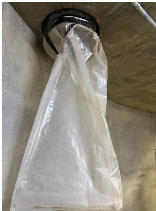
Figure 6 - 225 Lower Floor Air Intake (Dry Pit)
