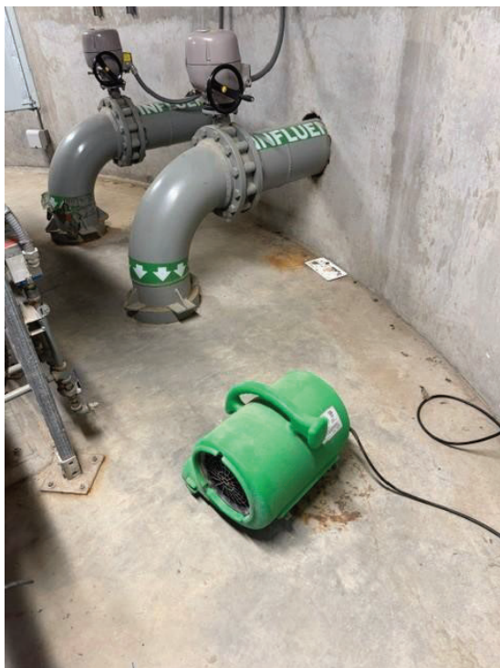
Figure 5- 225W Lower Floor Supplemental Ventilation
