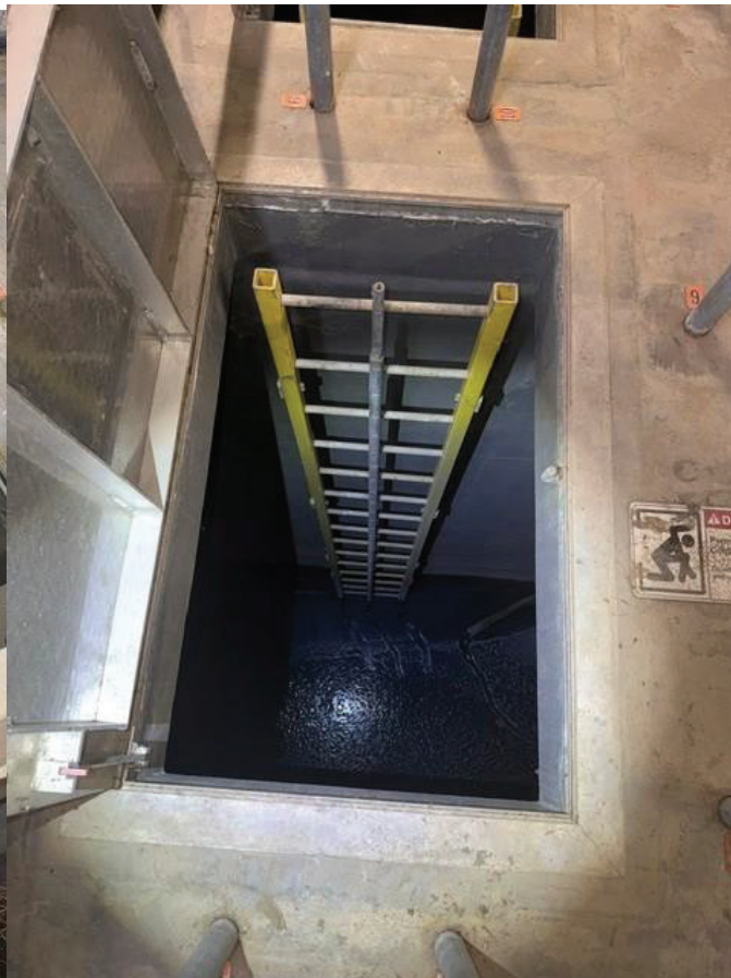
Figure 4 – 225W North Sump Tank
