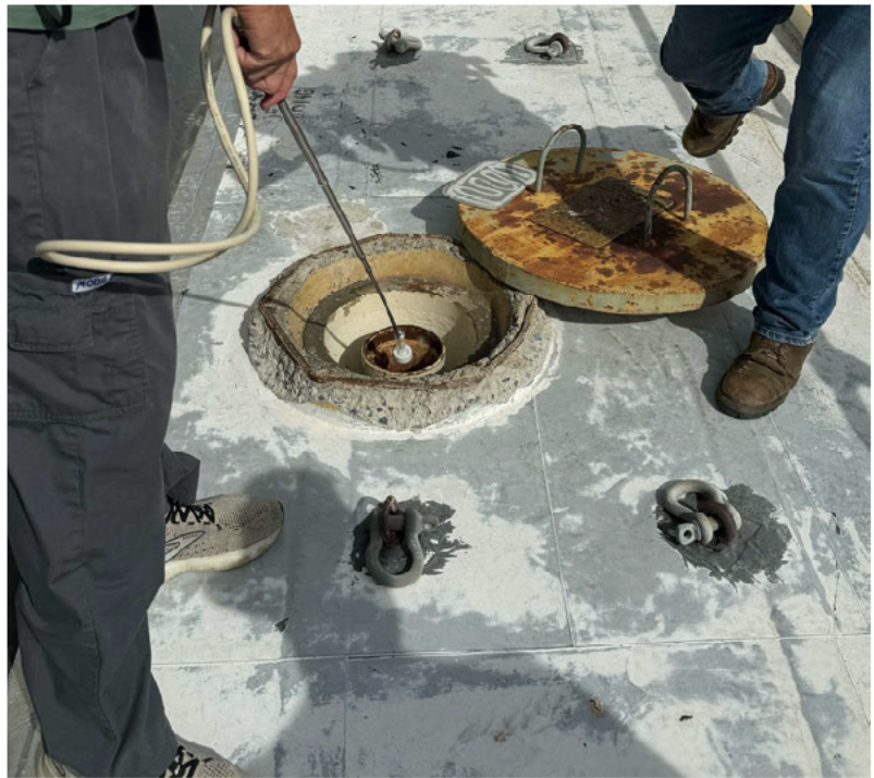
Picture 2-IHT Monitoring of Open Lid and Pipe Chamber
