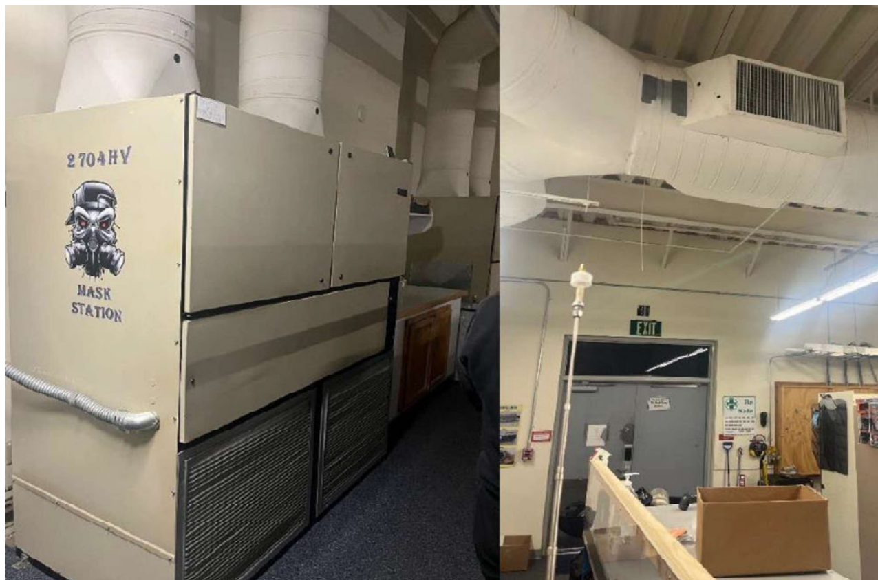
Figure 1: Room H105 RPE Issuing Station
