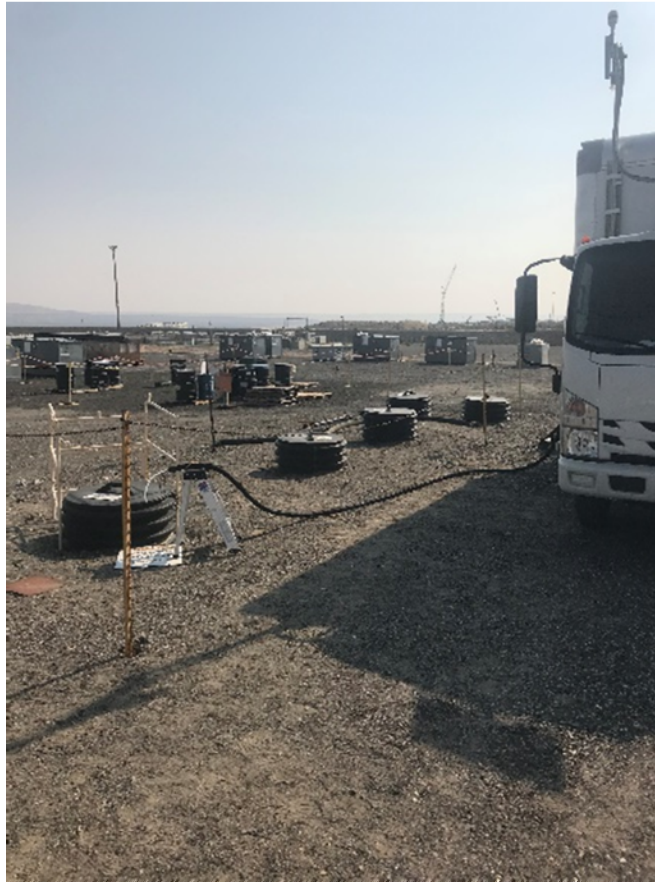
Figure 2-4. Septic Tank Monitoring.
