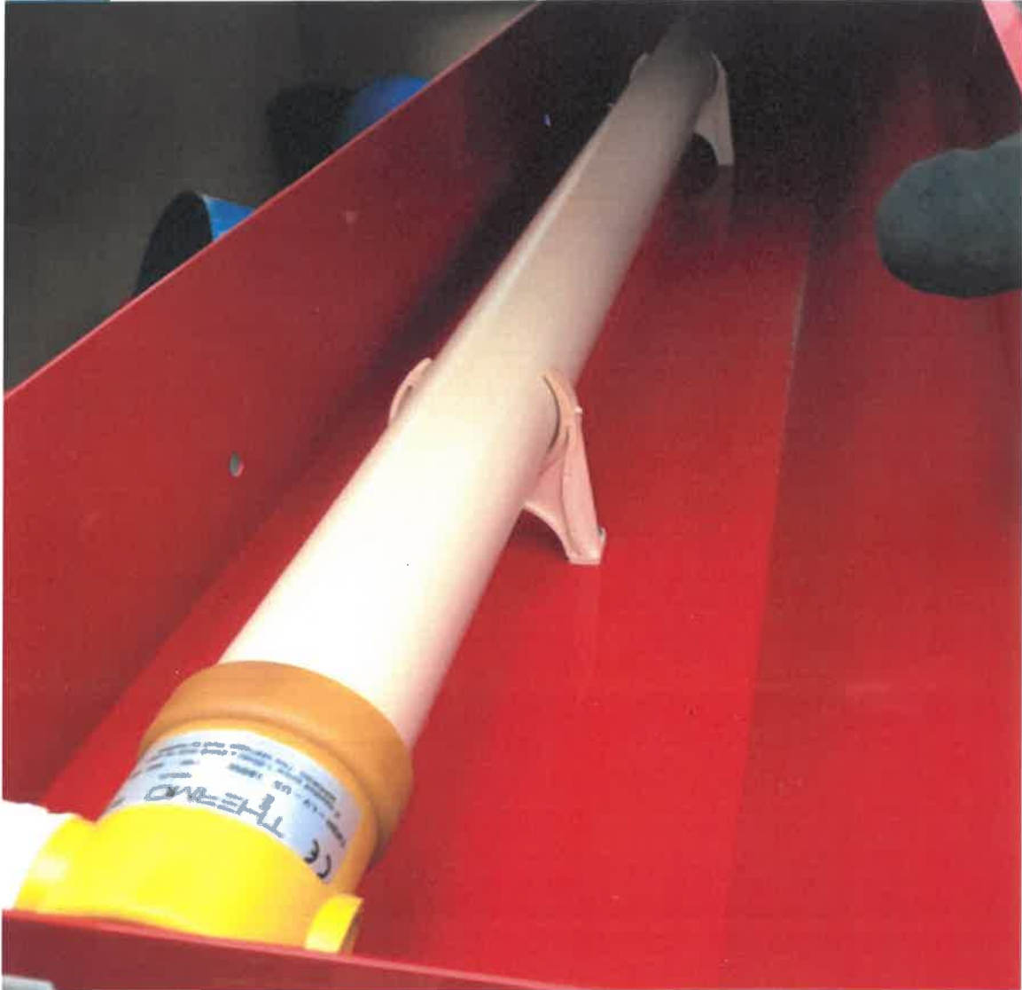
Figure 3: Heating Assembly Located Inside of KNAACK Job Box
