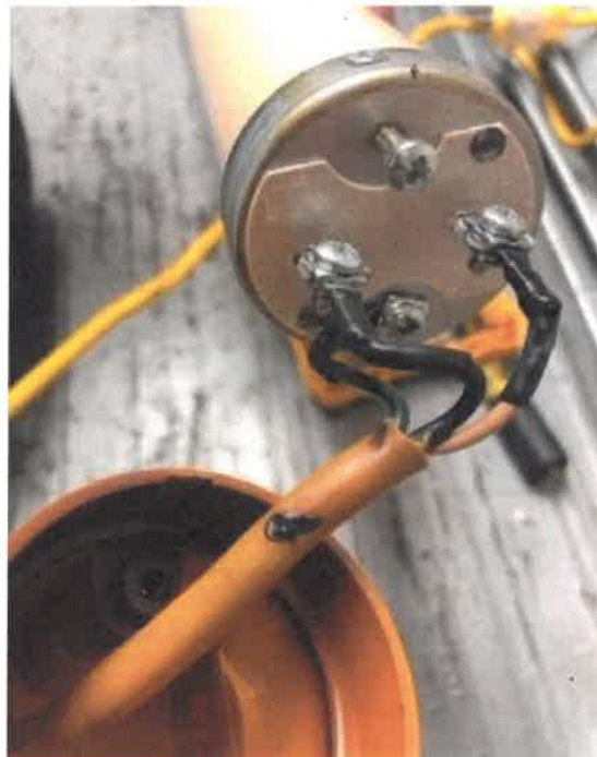
Figure 1: Partially Melted Outer Cord Covering
