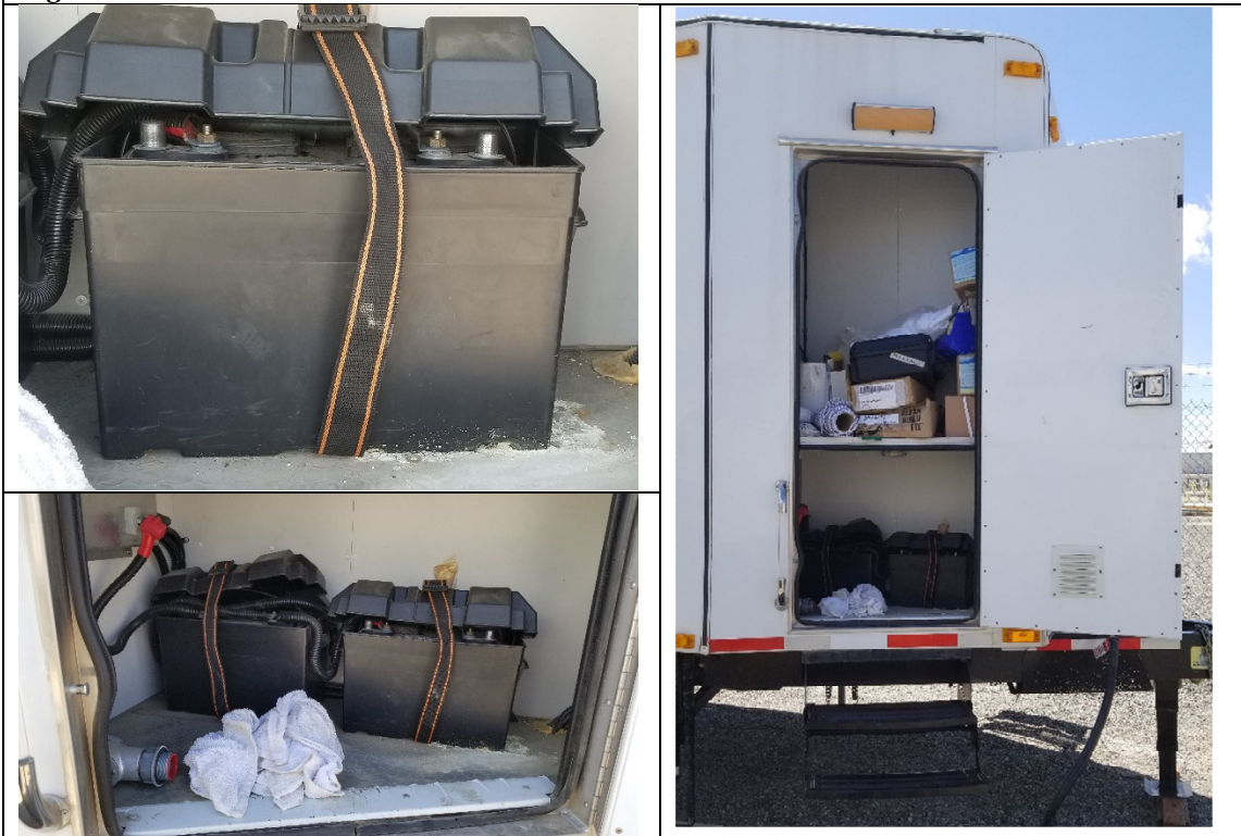
Figure 3. Corroded Batteries Found in the UT Trailer
