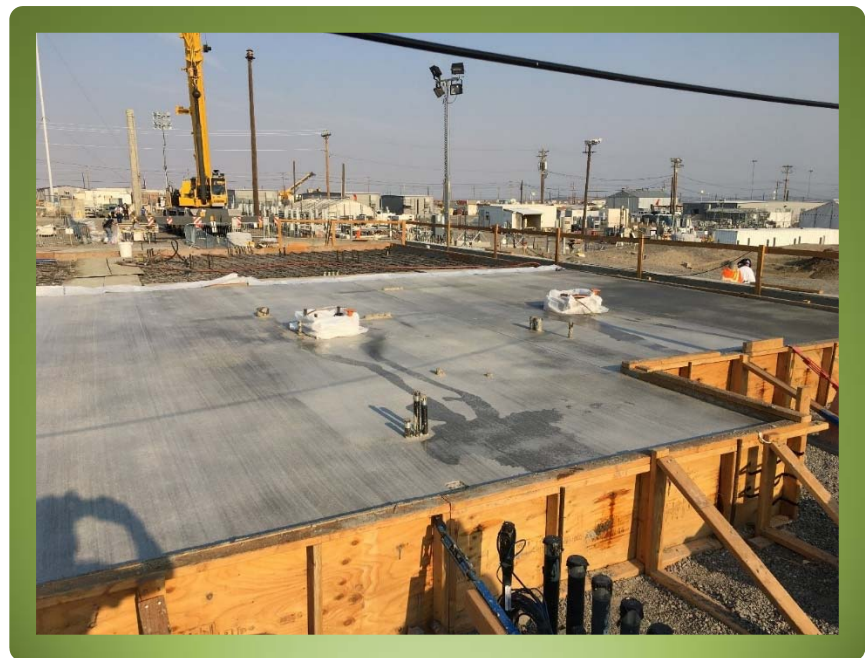
Figure 2. Completed Concrete Pour for east side of A-Farm Exhauster Slab (Photo courtesy of M. Allen)
