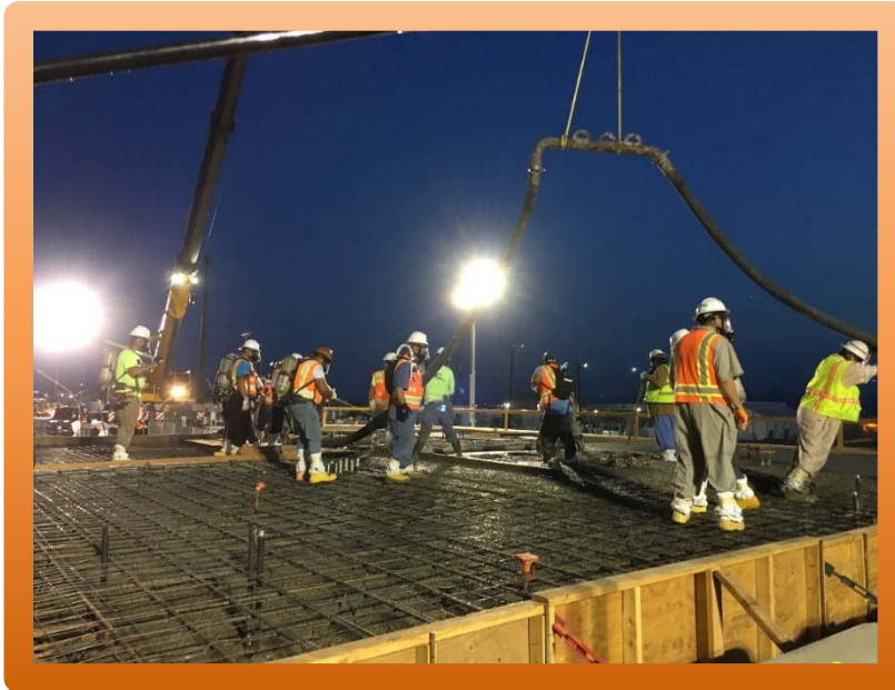
Figure 1. Installing Rebar and Pouring Concrete for A-Farm Exhauster Slab. (Photo courtesy of M. Allen)
