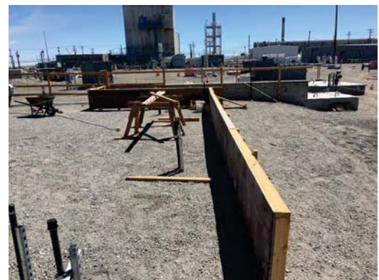
Figure 3. Exhauster Slab Concrete Forms for A Farm Exhauster (Photo courtesy M. Allen.)
