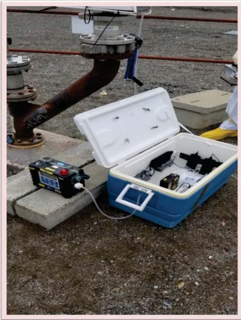
Figure 5. C 2 Sense® System Installed at A-103 Passive Breather Filter (Photo courtesy of E. Morrey.)
