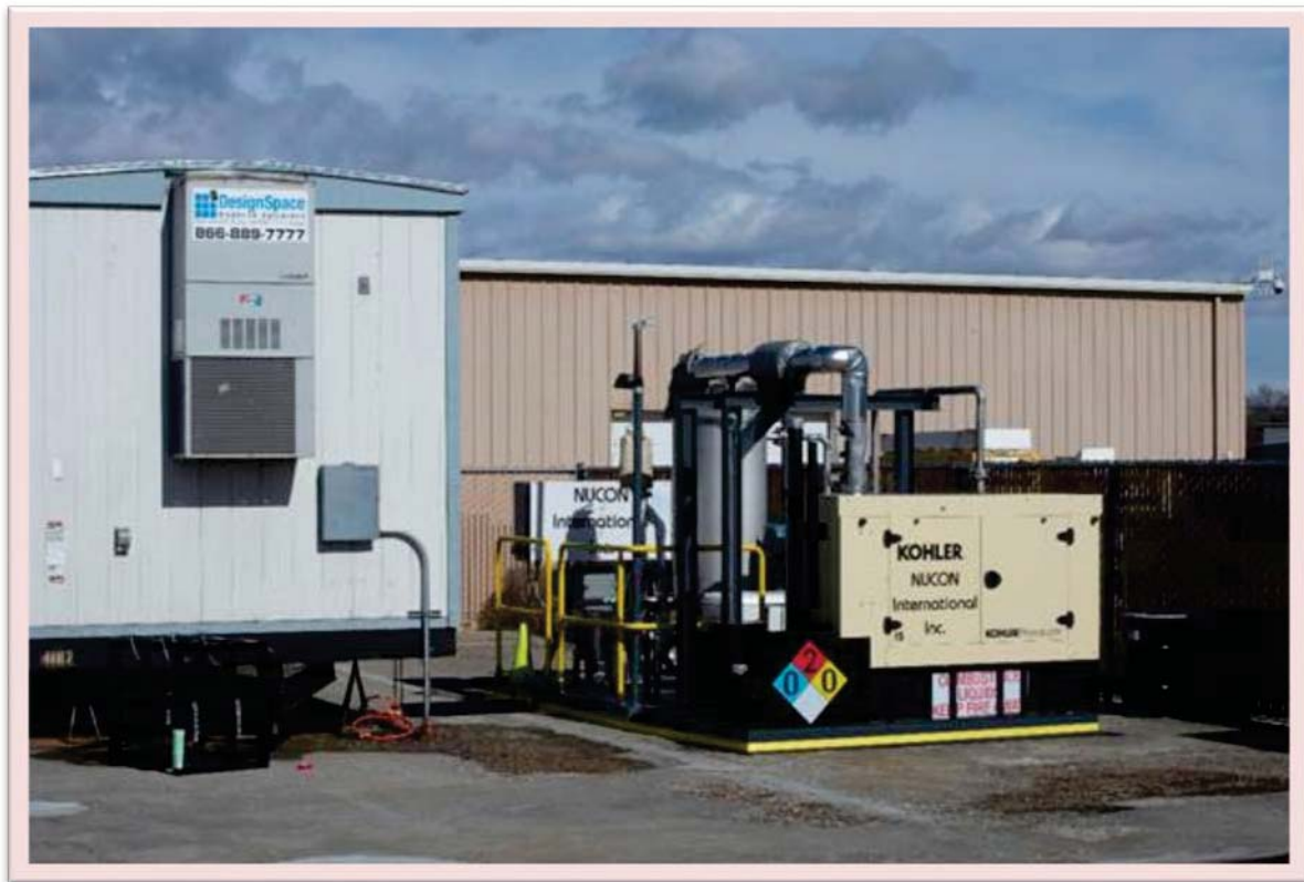
Figure 4. NUCON® Vapor Abatement Unit and Instrumentation Trailer
