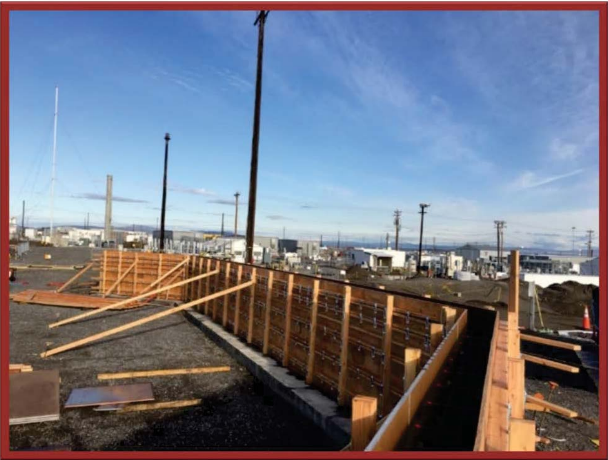
Figure 2. Pictured is an A Farm Exhauster Retaining Wall. The rebar and forms have been installed and are awaiting the concrete. For more, see KPP 4, Engineering Controls. (Photo courtesy of M. Allen.)
