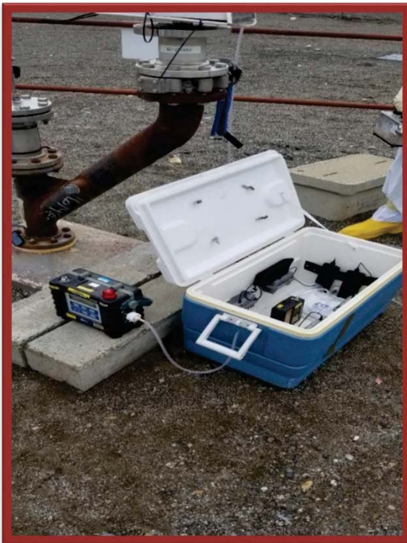
Figure 5. C 2 Sense® System Installed at A-103 Passive Breather Filter (Photo courtesy of E. Morrey.)
