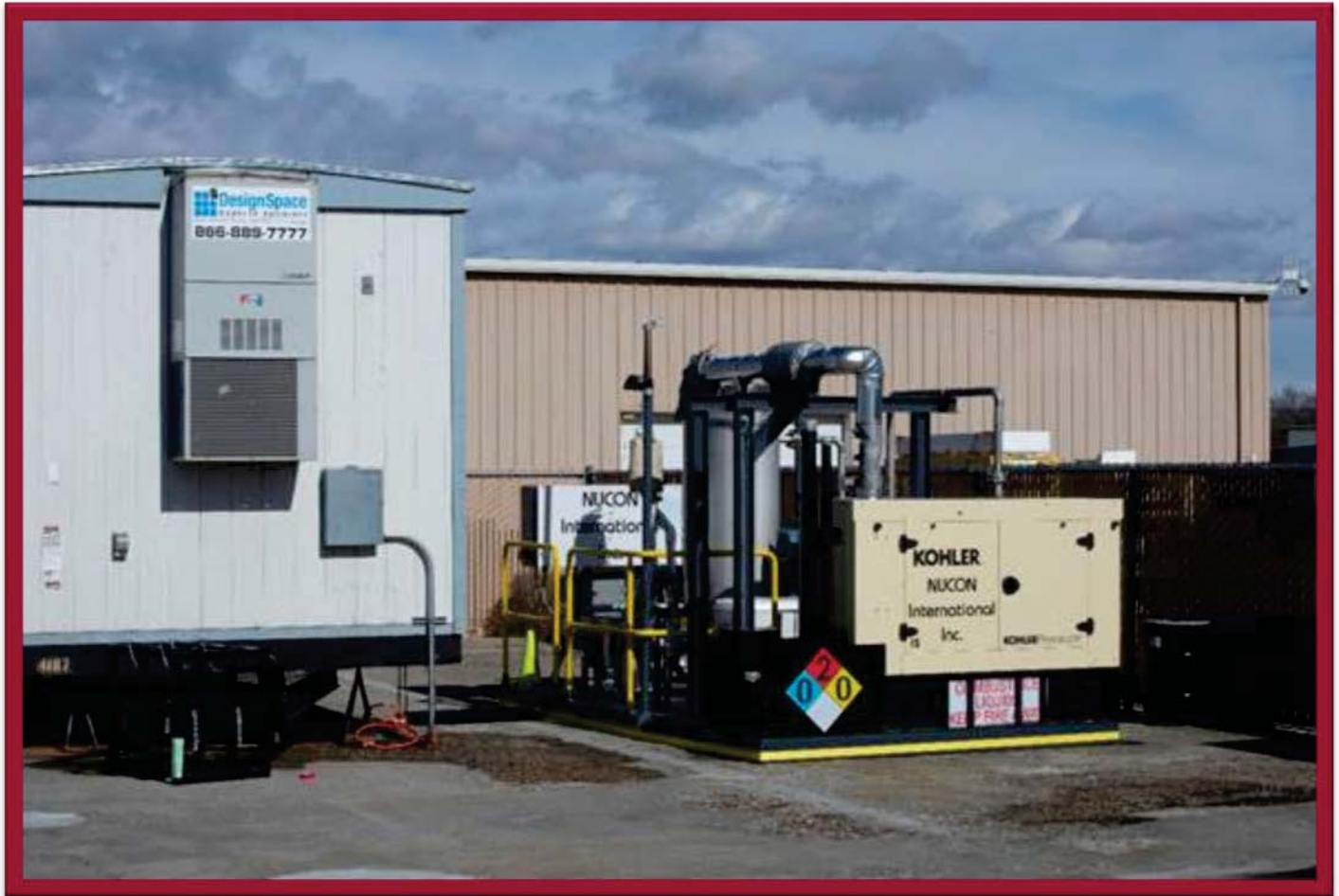
Figure 4. NUCON® Vapor Abatement Unit and Instrumentation Trailer
