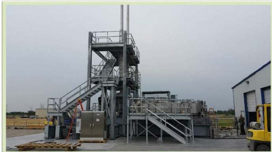
The A Farm Exhauster, fabricated in FY2017, is currently located in Blackfoot, Idaho, at the manufacturer's facility. Projects is working on the ducting installation and pad design/installation preceding the exhauster's installation. (Picture courtesy Mark A.) More in KPP 4 .
