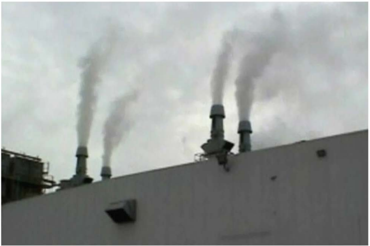
Strobic Air Ventilators
