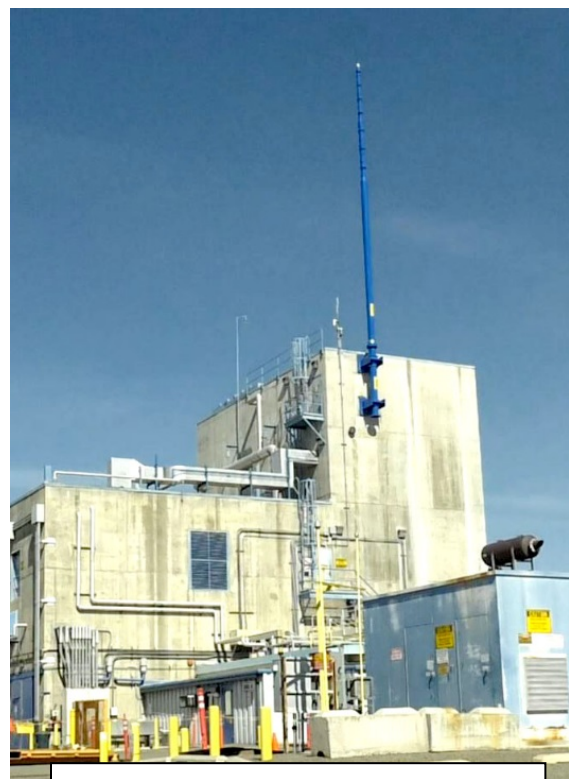
New ventilation stack on the 242-A Evaporator is 111 feet above ground.
